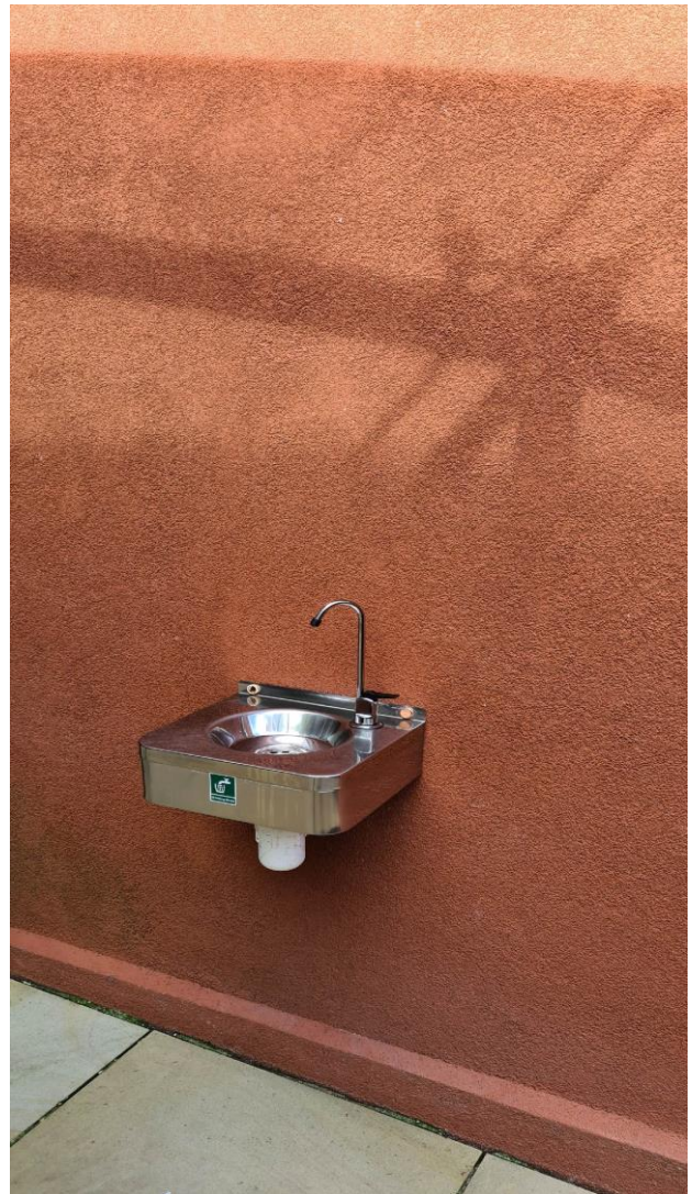
Drinking Water Fountain
